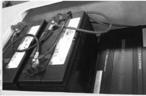
Figure 1. Battery and converter.
