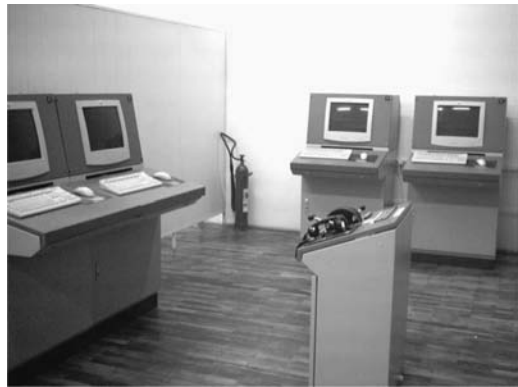
Figure 3. Local Control Room with 4 Local Operating Stations (LOS).
