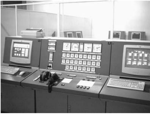
Figure 1. Engine control room.
